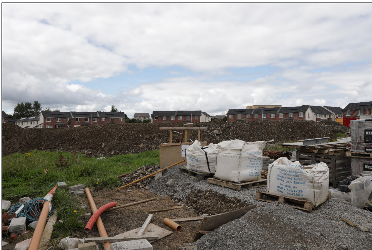
VIEW 13 – Proposed view from Phase 2 Dun Rioga across central open space (Under construction)
